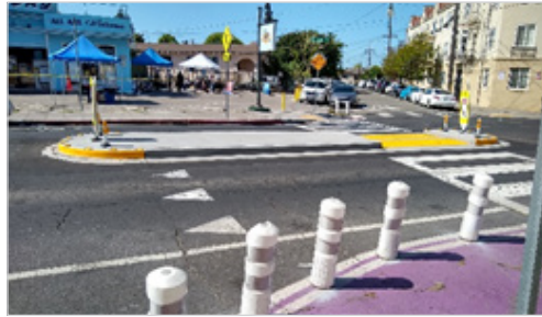
Safety island and modular curb for the City of Oakland's Slow Streets.
