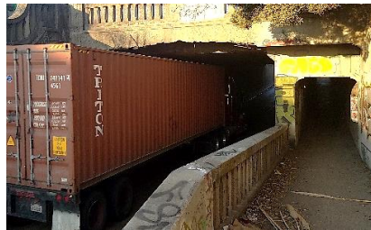
Existing multi-use path and damage to the 7th Street underpass.
