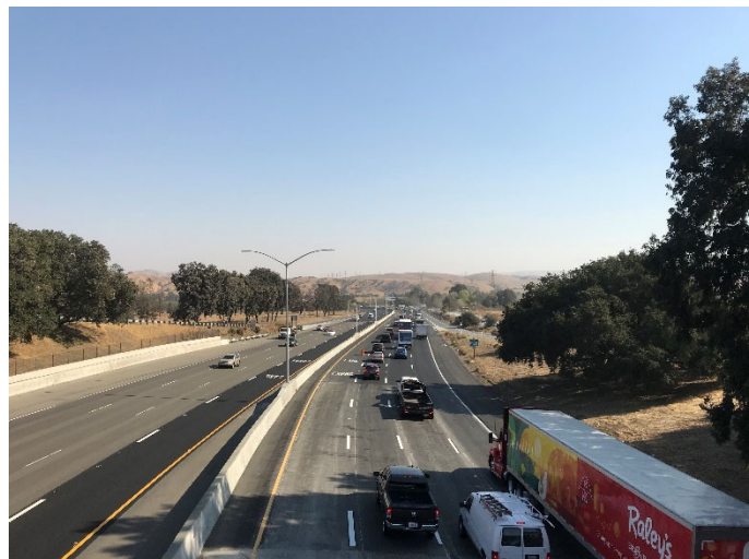
The existing I-680 Sunol Southbound Express Lane was converted from restricted to continuous access in October 2020 as part of the capital project construction.
