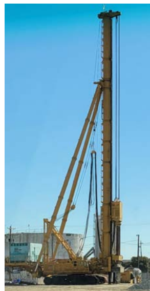
The now assembled "Big Bird," digs deep holes to insert steel reinforcement and concrete piles into the ground.
