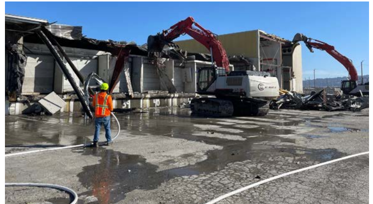
Demolition of the old PCC Logistics building at the Port of Oakland is making way for the new 7th Street roadway
