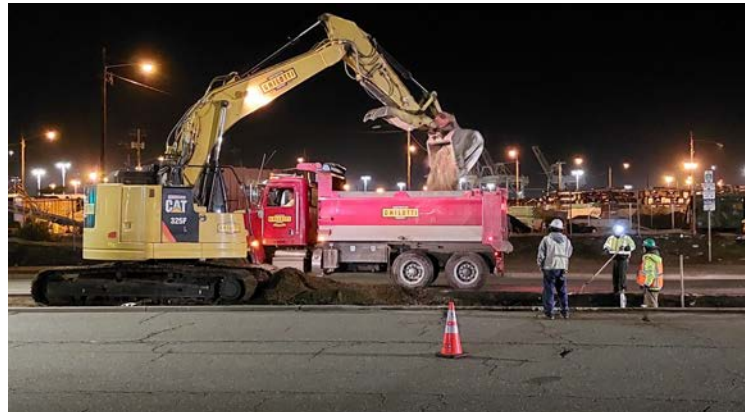
An excavator and dump truck are used to install and connect new storm drainpipes.
