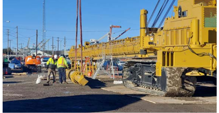
Prior to construction, a huge drill rig nicknamed "Big Bird" is being assembled.
