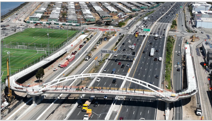
Bicycle and pedestrian overcrossing that is Phase 1 of the I-80 Gilman Interchange Improvements project.
